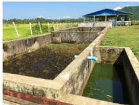
Figure 8. Front view of Sludge Treatment Systems in Sin Tet Maw, Pauktaw
